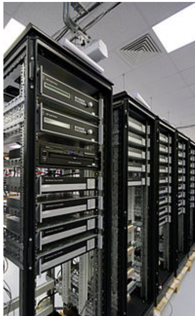
Public address system consisting of amplifiers, mixers, and routers for a major international airport
