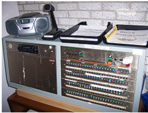
Public address system in an old high school
